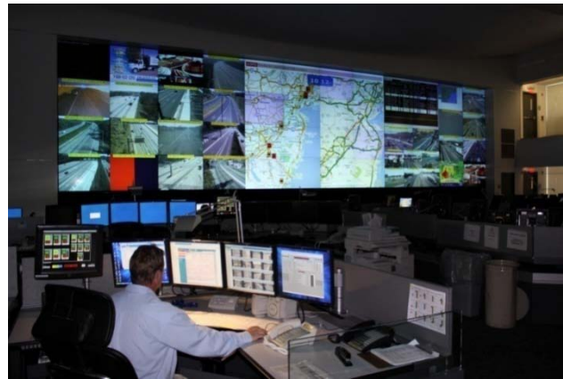
Figure 2.4: View from inside the NJDOT TMC
